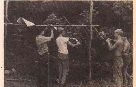
The lean-to takes shape slowly but surely. It leaked like a sieve!
